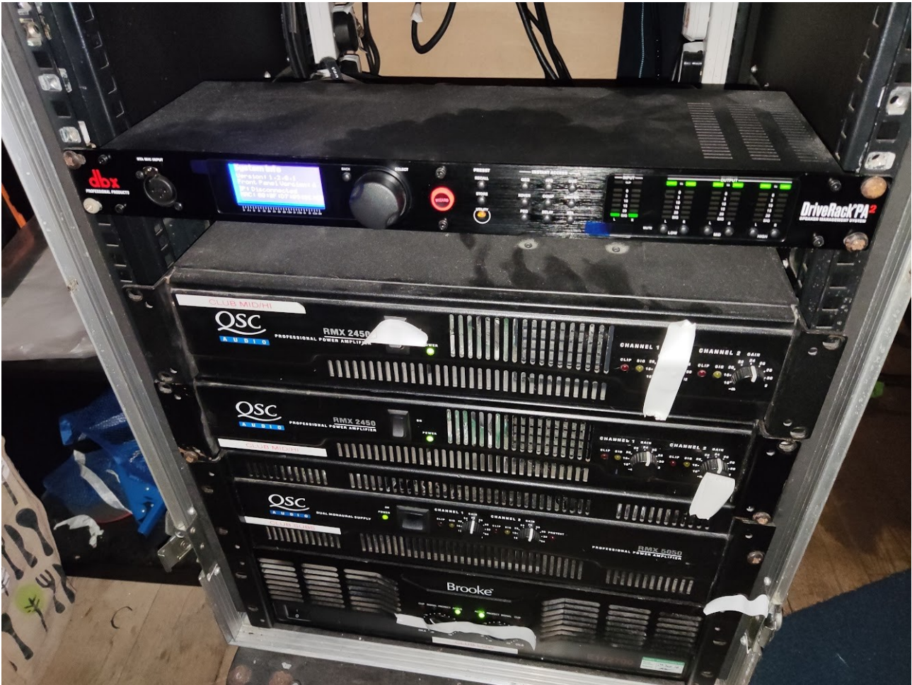
Figure 1: Equipment rack with dbx DriveRackPA2 (the limiter) at the top of the rack
